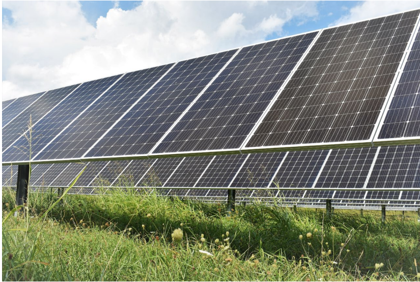
2.7 Megawatts of Solar
