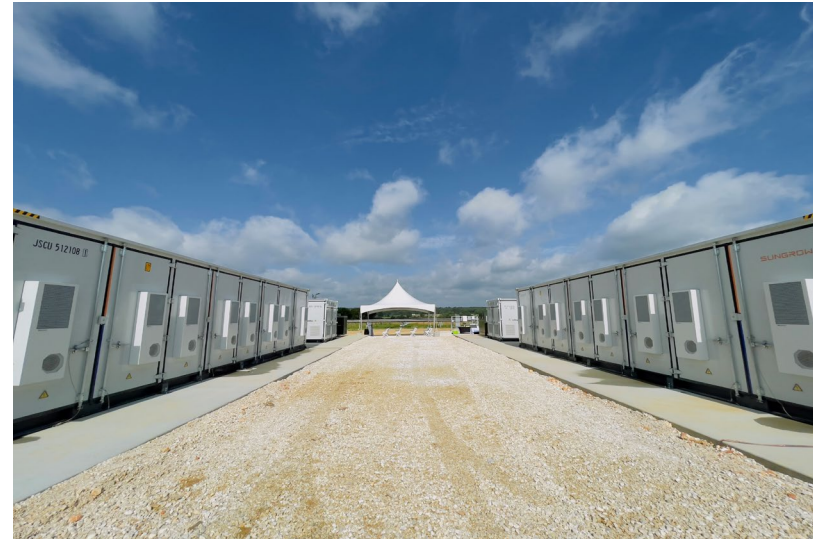
7 Megawatts of Energy Storage
